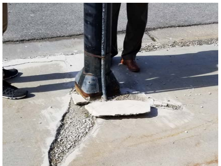
Figure 3.05 - Examples of accessibility challenges in Downtown Gardner
