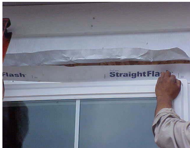
Flashing tape across top of window with housewrap folded down over it
