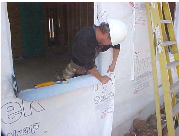
Apply sill flashing across bottom of sill and approximately 8 inches up each side
