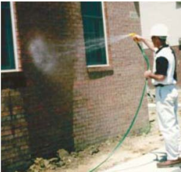
In this hose test, water penetrated this brick veneer in less than one minute
