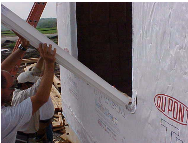
Set the bottom of the window on shims and tilt into place
