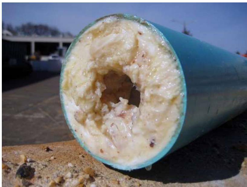
EXAMPLE: Severely plugged PVC sewer line by grease.
