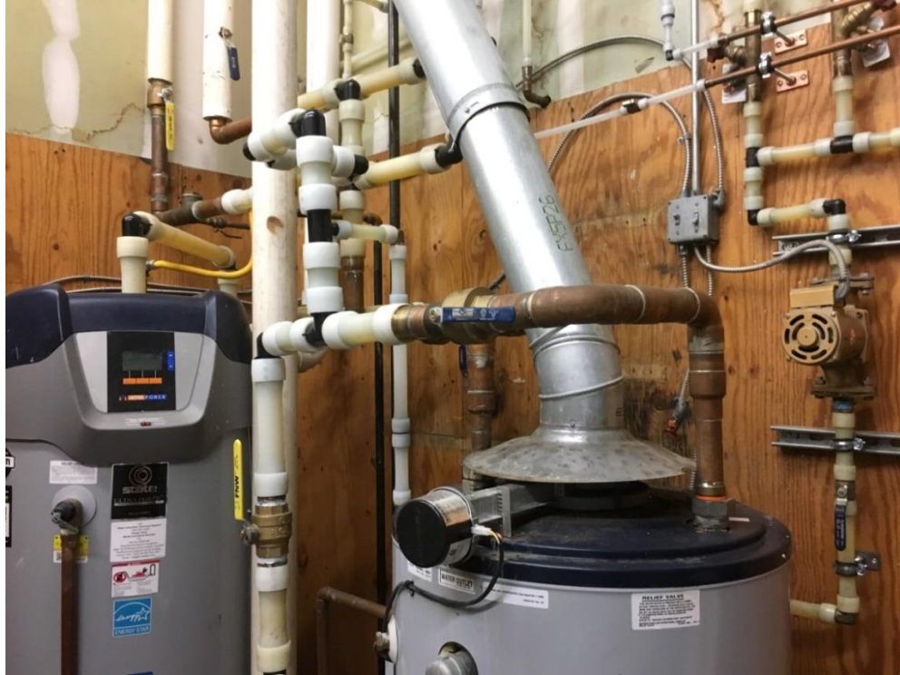
Photograph 10- Repairs to plumbing system from copper pipe electrolysis condition.
