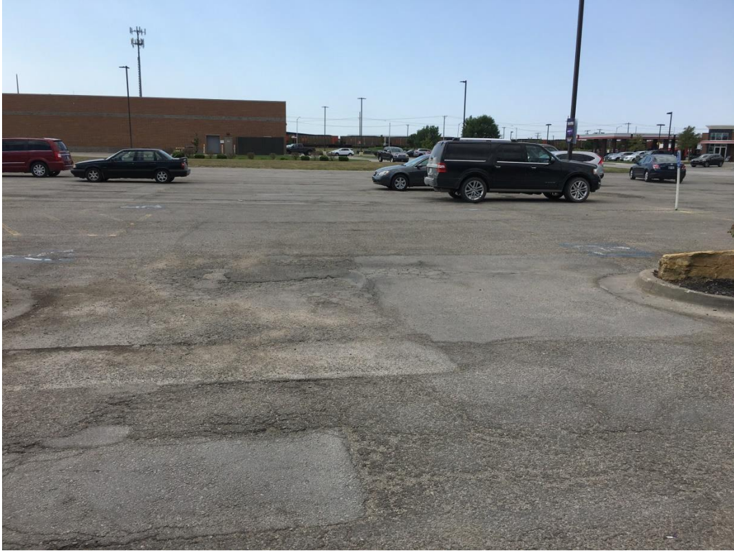
Photograph 37- Deterioration of site improvements.
