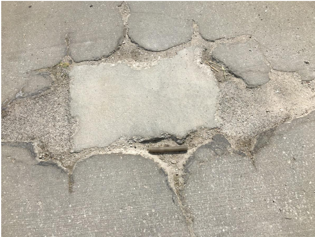
Photograph 34- Deterioration of site improvements.
