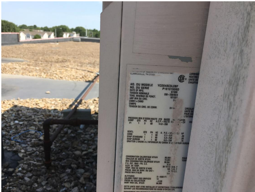
Photograph 4- 830 E Main Street, roof top units (RTU's) label shows they were manufactured in 1999 and are over 19 years old. The fins also show hail damage that can restrict airflow.
