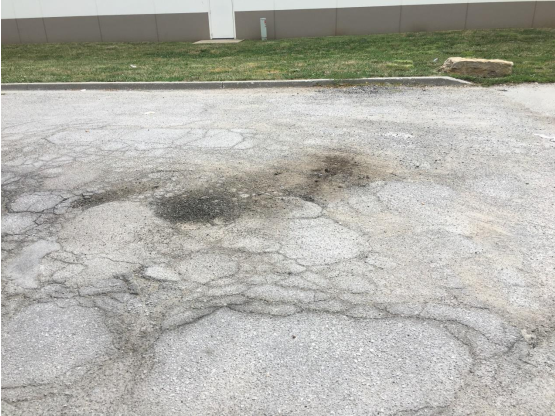
Photograph 35- Deterioration of site improvements.
