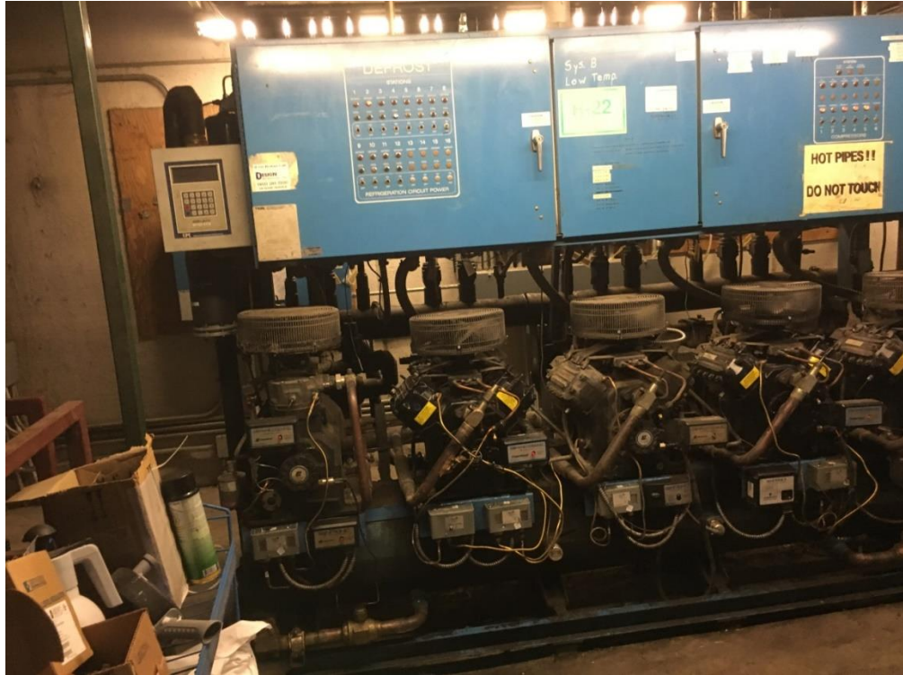
Photograph 5- Expensive infrastructure like refrigeration and HVAC are in place, and are at the end of their life expectancy, and not as efficient as modern equipment.
