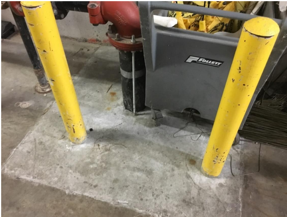
Photograph 11- Repairs to plumbing system from copper pipe electrolysis condition, the main water line was deteriorated.
