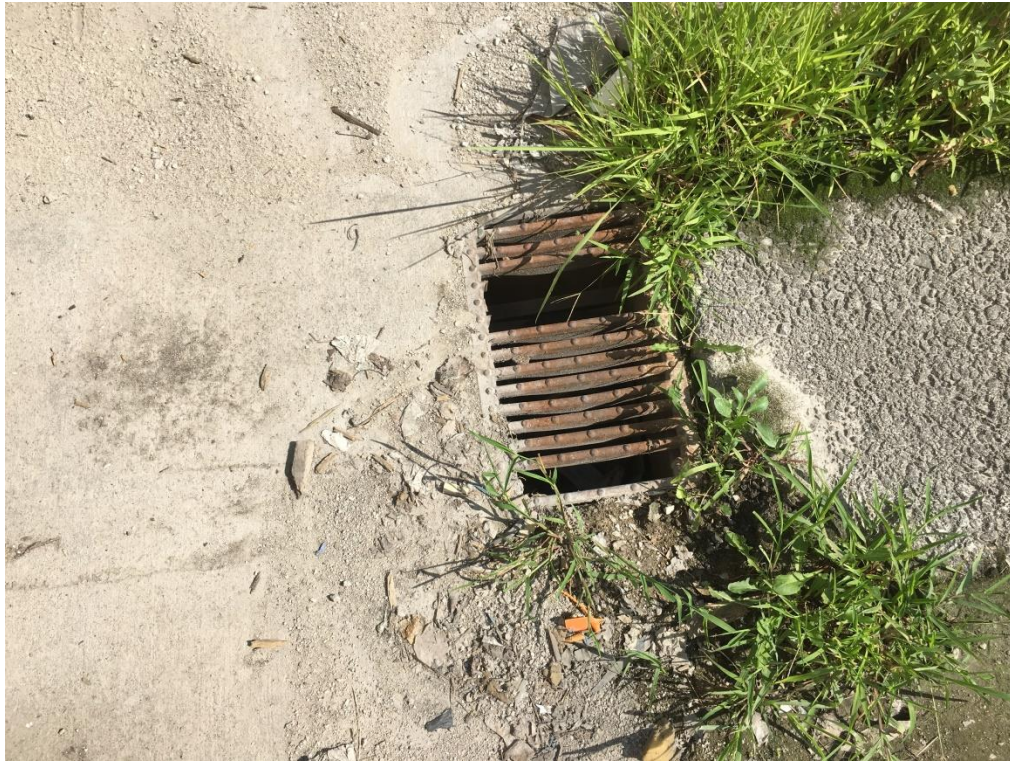
Photograph 28- Location Lot 5, Broken grate, potential tripping hazard.
