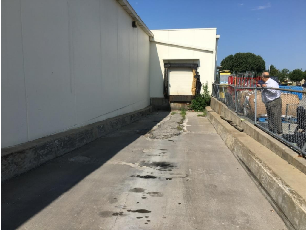
Photograph 41- Location Lot 5- Trees growing at side of building.
