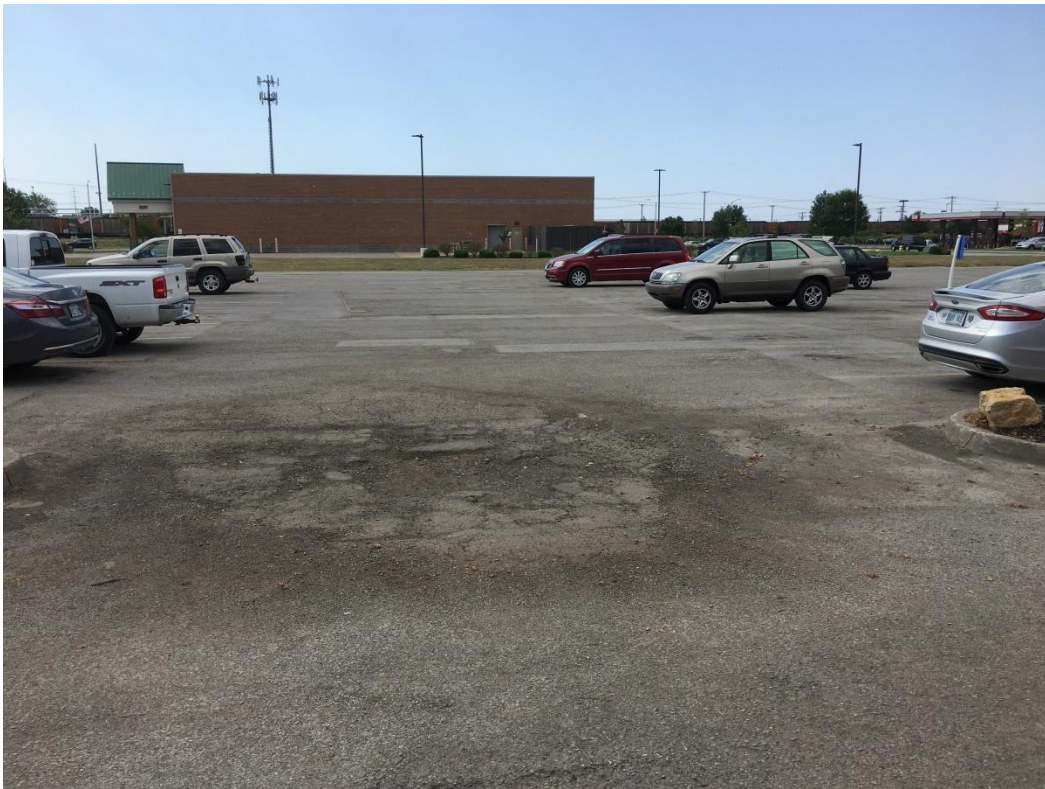
Photograph 36- Deterioration of site improvements.
