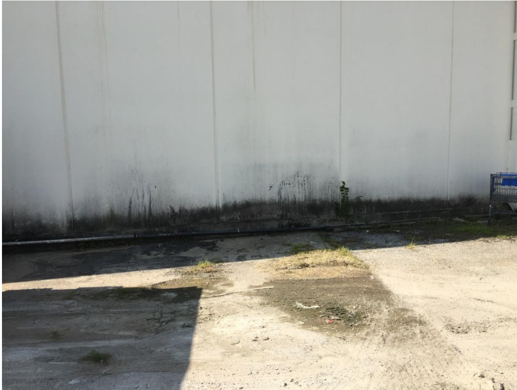
Photograph 12- Lot 5- building façade deterioration in rear dock loading area.
