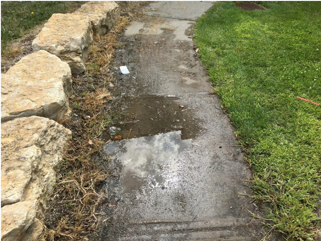
Photograph 42- Standing Water on Lot 3.
