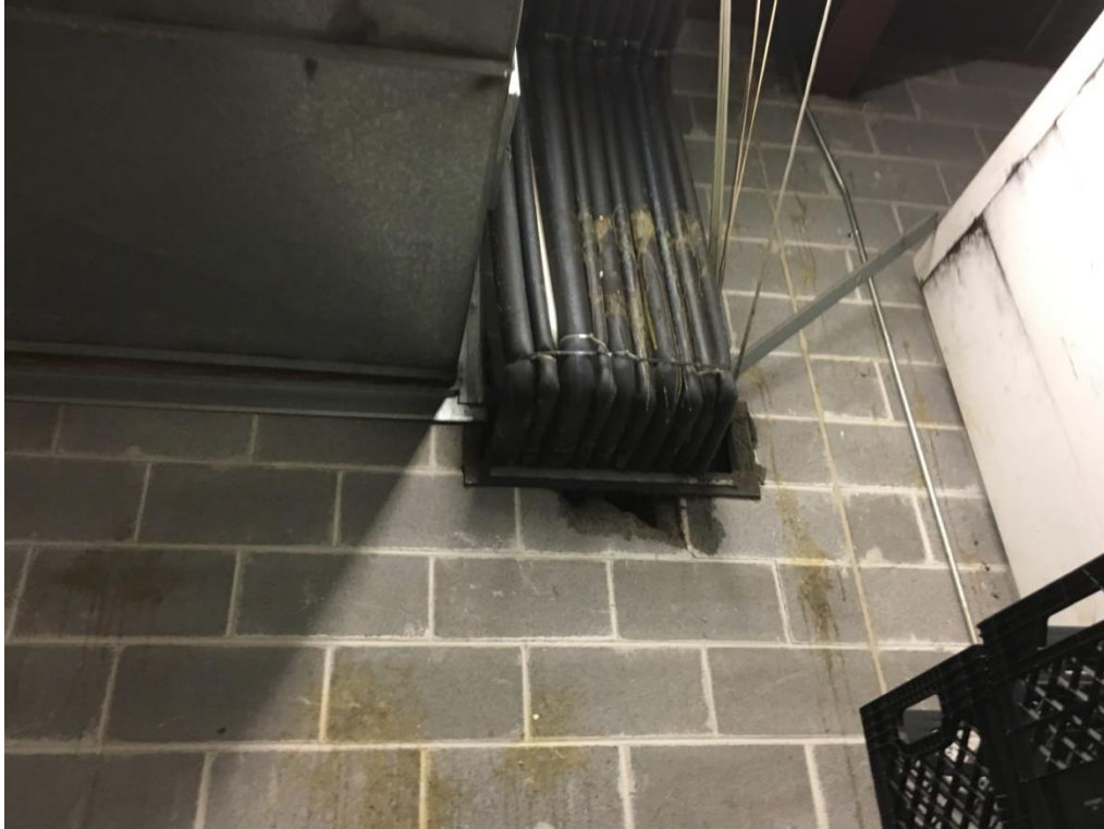
Photograph 7- Expensive infrastructure like refrigeration and HVAC are in place, and require more maintenance than modern equipment.
