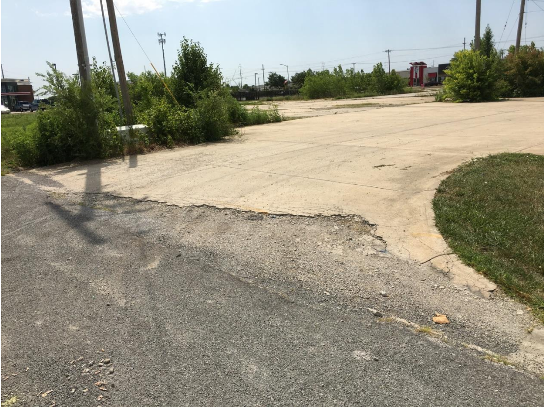
Photograph 39- Deterioration of site improvements.
