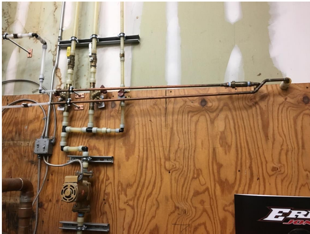
Photograph 9- Repairs to plumbing system from copper pipe electrolysis condition.
