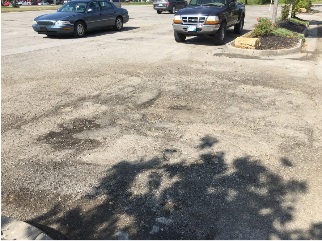
Photograph 33- Deterioration of site improvements.
