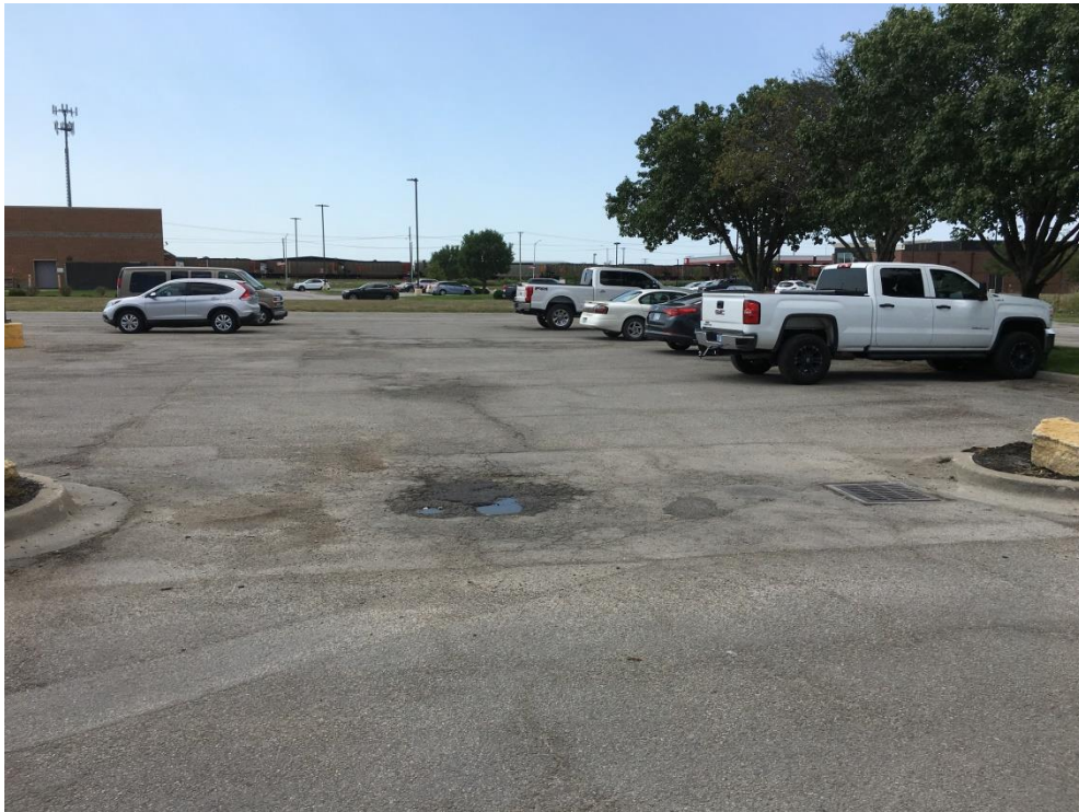
Photograph 29- Location Lot 5- Large pot holes in pavement, potential tripping hazard.
