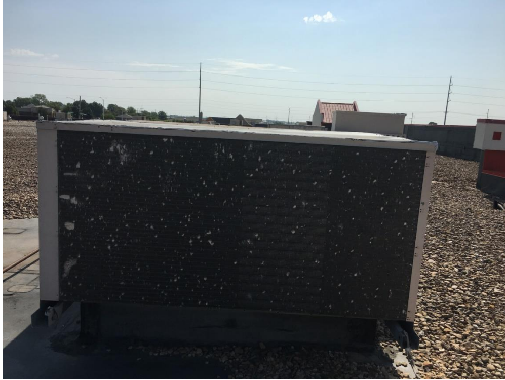
Photograph 3- Roof of 830 E Main Street, roof top units (RTU's) was manufactured in 1999 and is over 19 years old. The fins also show hail damage that can restrict airflow.
