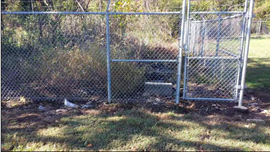
Figure A16: Decant Drain to Surface (South Edge of Property) (Facing S), 10/07/2016
