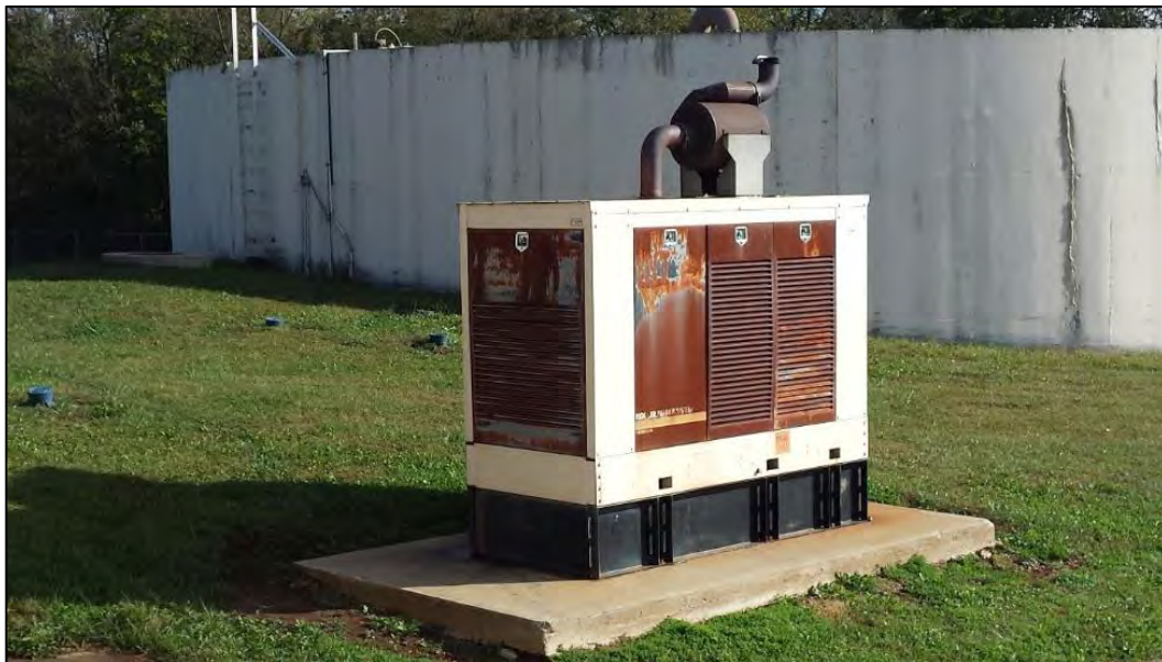
Figure A25: Generator to East of Building (Facing NE), 10/07/2016
