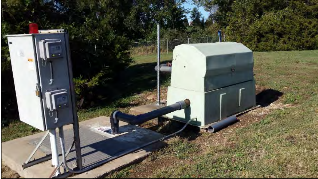
Figure A12: Sludge Pump (South Region of Property), 10/07/2016
