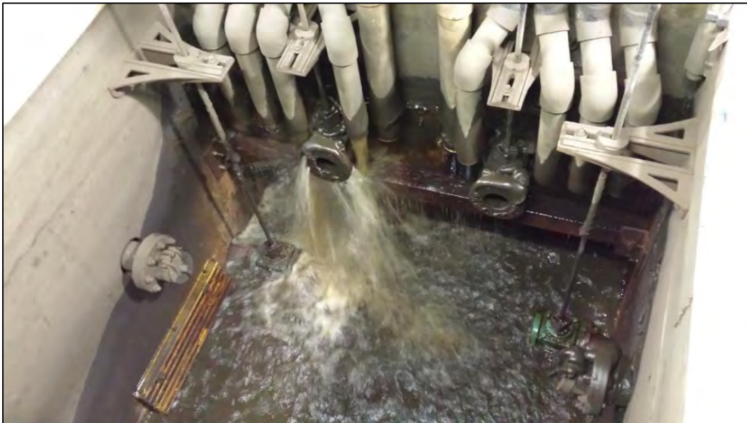
Figure A11: Clarifier Blowdown (Basement Floor), 10/07/2016
