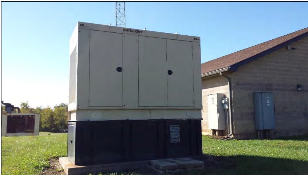
Figure A27: Generator to Northeast of Buildings (Facing S), 10/07/2016
