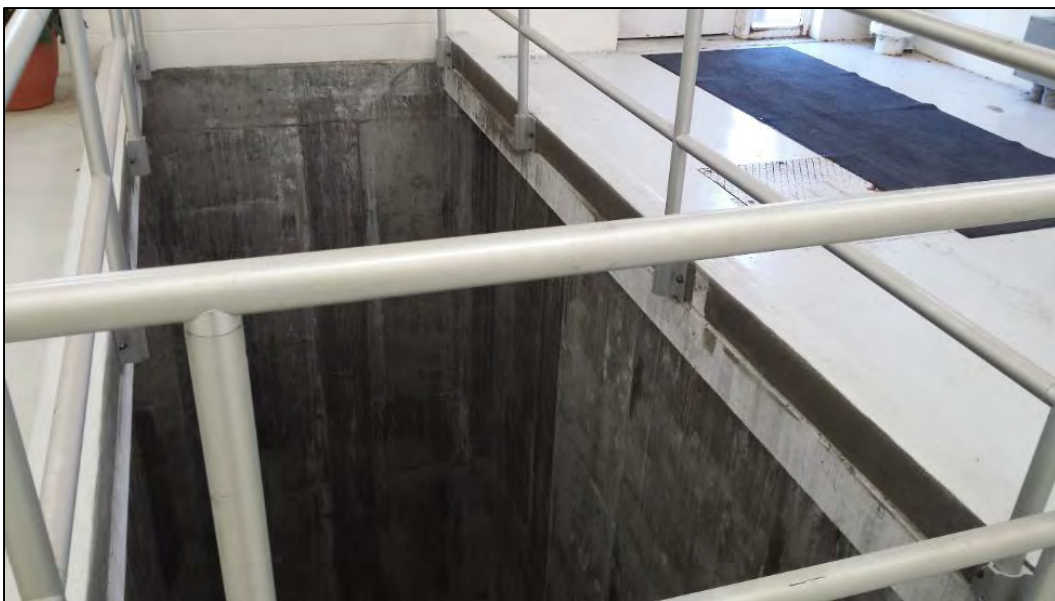
Figure A7: Unused Filter Cell, 10/07/2016
