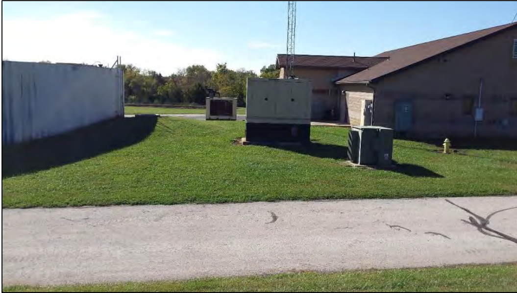
Figure A26: Generator to Northeast of Buildings (Facing S), 10/07/2016
