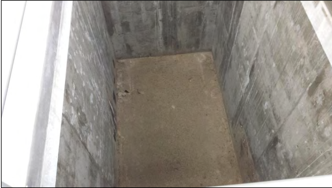
Figure A6: Unused Filter Cell, 10/07/2016
