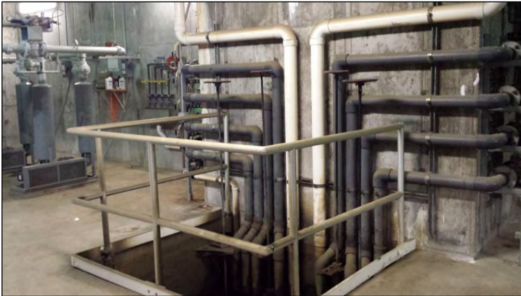
Figure A10: Clarifier Blowdown (Basement Floor), 10/07/2016
