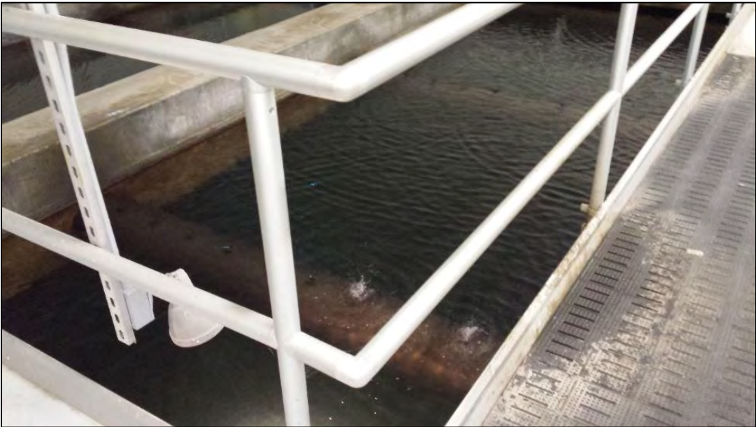
Figure A2: Pulsating Clarifier and Launders, 10/07/2016
