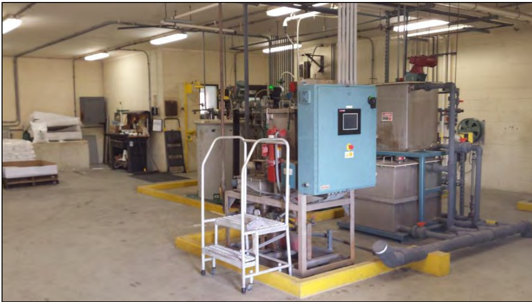
Figure A22: Polymer Storage and Feed System, 10/07/2016
