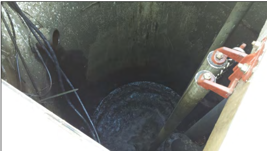
Figure A13: Sludge Pump (South Region of Property), 10/07/2016
