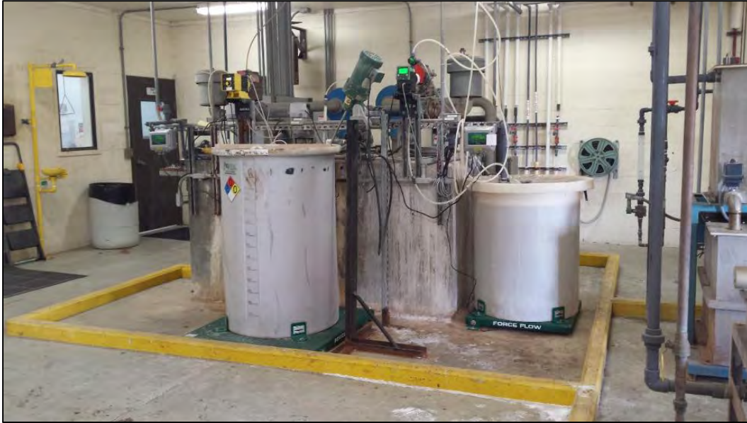
Figure A23: Polymer Storage and Feed System, 10/07/2016
