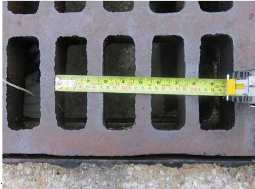
Grate openings 2"; replace with compliant models (gaps 1/2" max)
