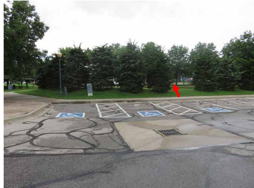
View of Aquatic Center Accessible Parking that can serve Cornerstone Curb cut(s) needed to connect accessible route Red Arrow: Location of same option for route to amphitheater
