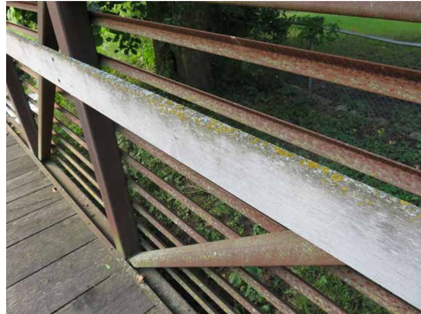
Provide compliant handrails and ensure effective edge protection. Handrails may be mounted to existing wood surface (34-38" ht.)
