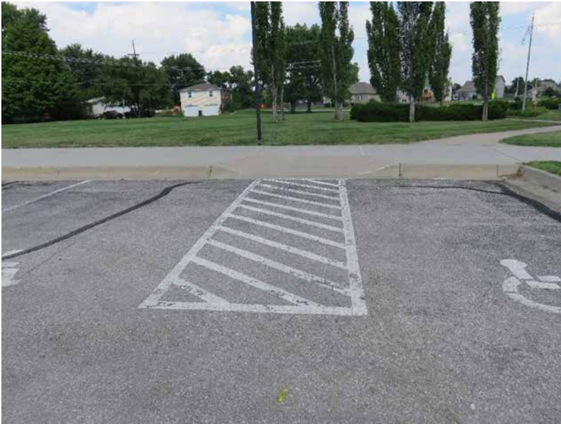
Parking spaces needing accessible signage Curb ramp slope should be mitigated in future alteration work
