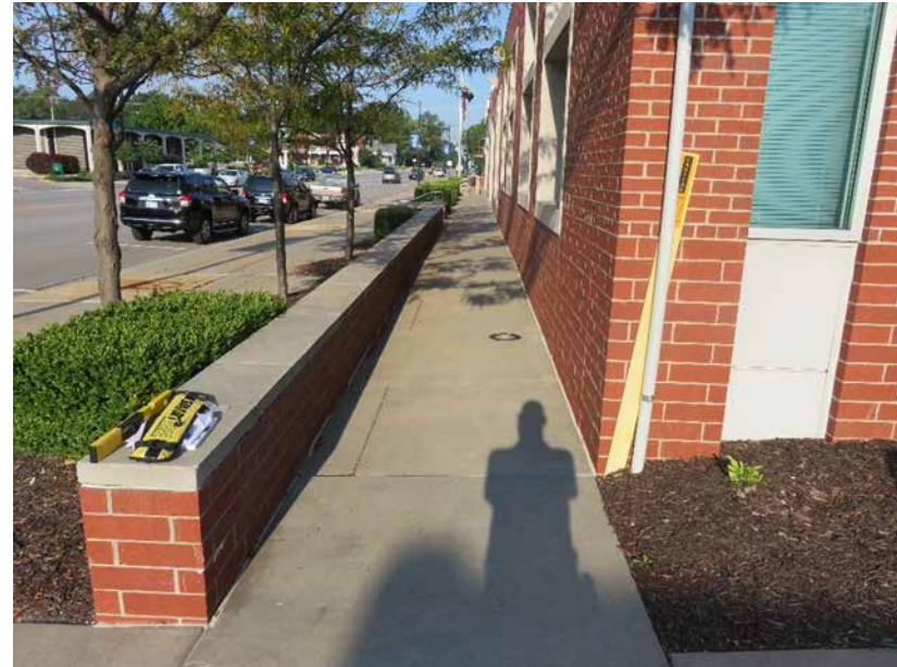
Cross slope and slope issues throughout turn compromise compliance
