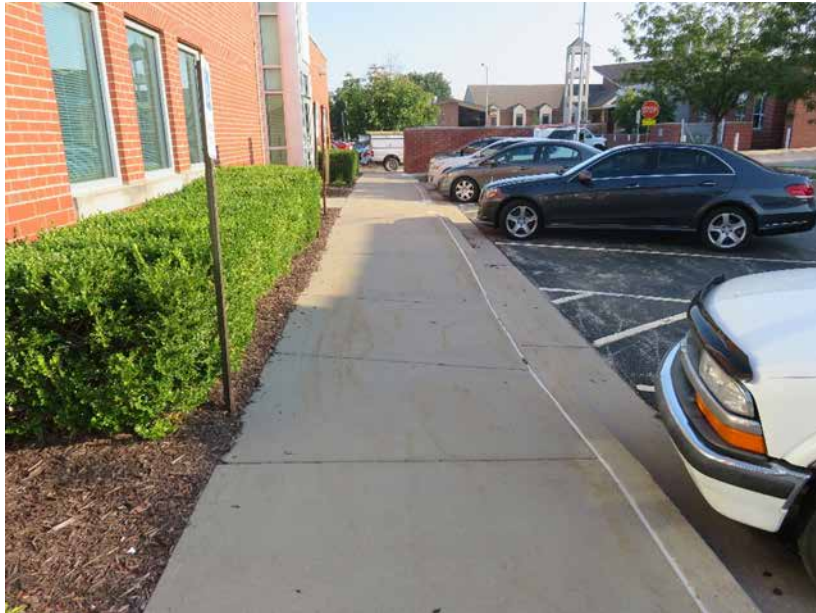
Curb ramp does not provide landing at top
