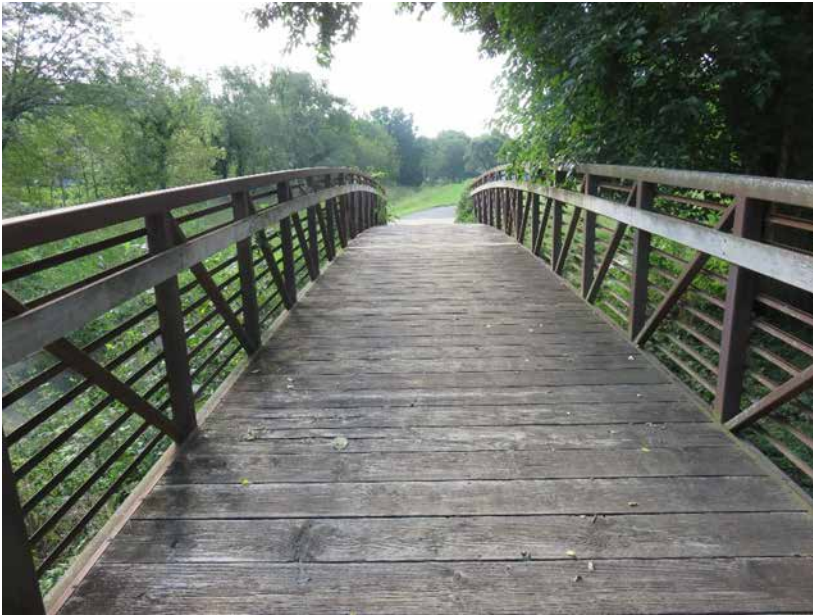
Bridge has ramp slope and requires compliant handrails.
