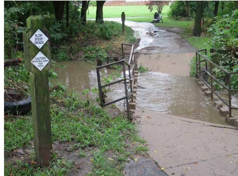
Recommend bolstering communication of danger on this route Enhance with larger signage providing better color contrast
