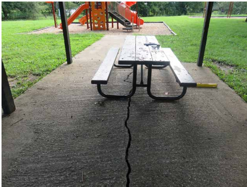
Large gap affecting slope of shelter ground surface.
