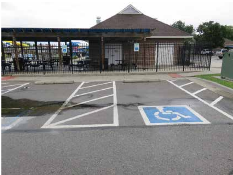
Address minor cross slope issues in spaces in future resurfacing
