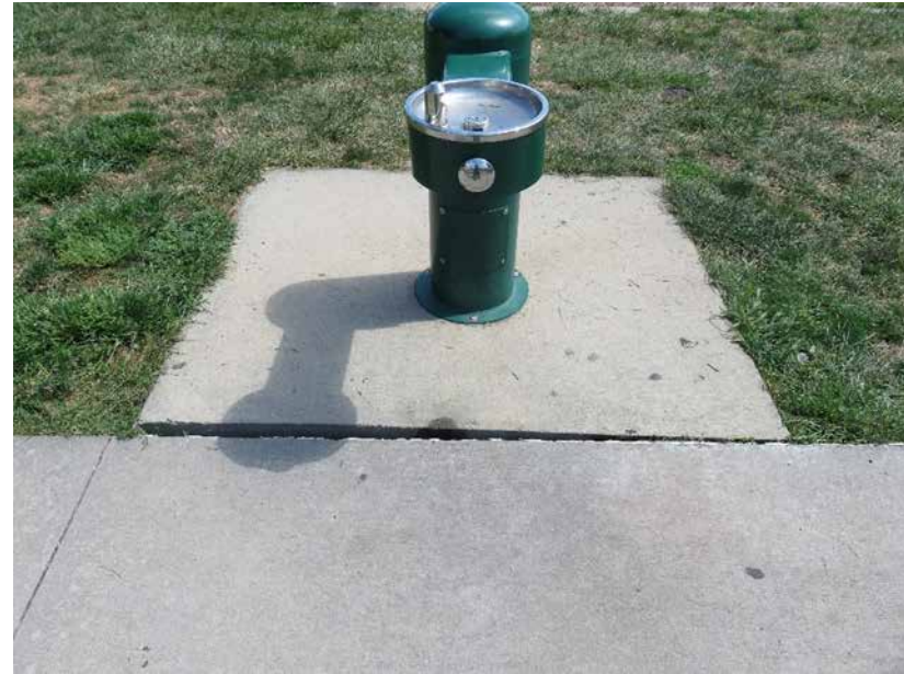
Changes in level/gaps: Settling between concrete areas
