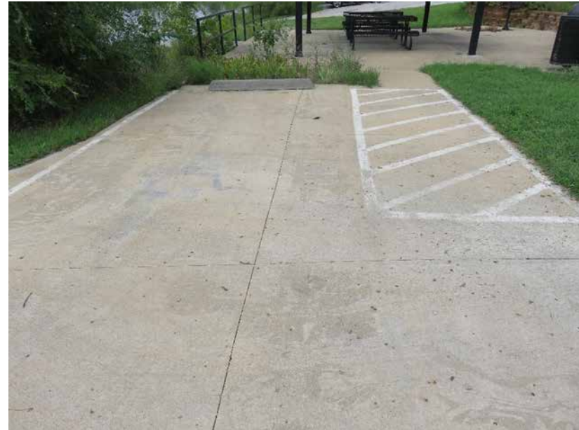
Provide accessible parking signage
