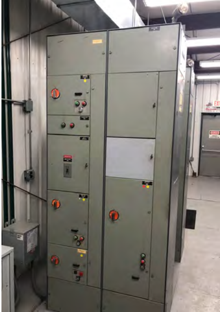
Motor Control Center # 2 Rear View
