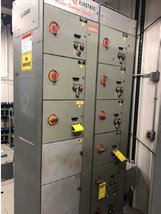
Motor Control Center #2 Front View
