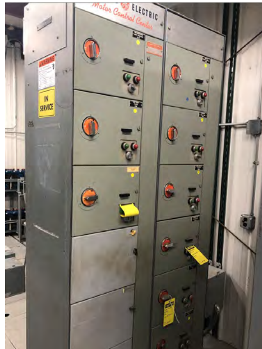
Motor Control Center #2 Front View
