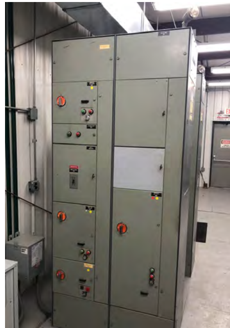
Motor Control Center # 2 Rear View
